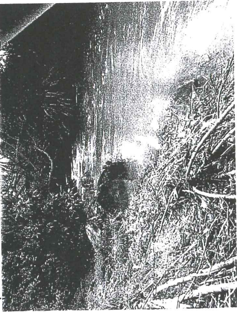
This is what is causing stormwater flooding in the Henderson Basin
