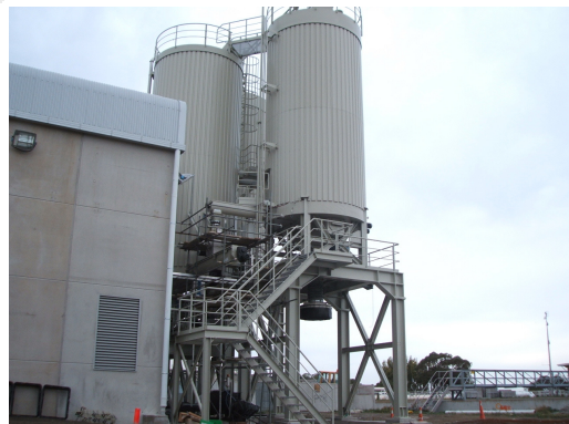
Biosolids Drying Facility at Bromley
