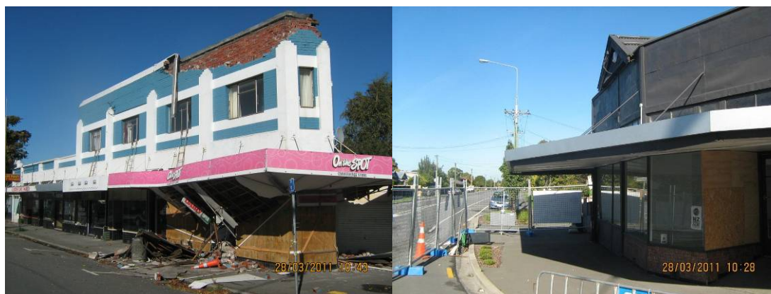
Figure 5. March 2011, damage to 299 Selwyn Street block
