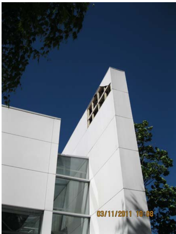
Typical damage to external cladding system.
