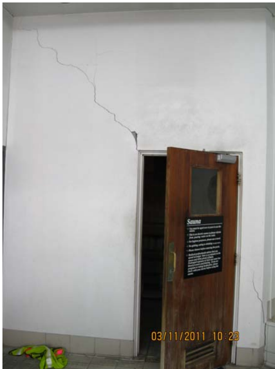
Damage to Blockwork walls (typical).
