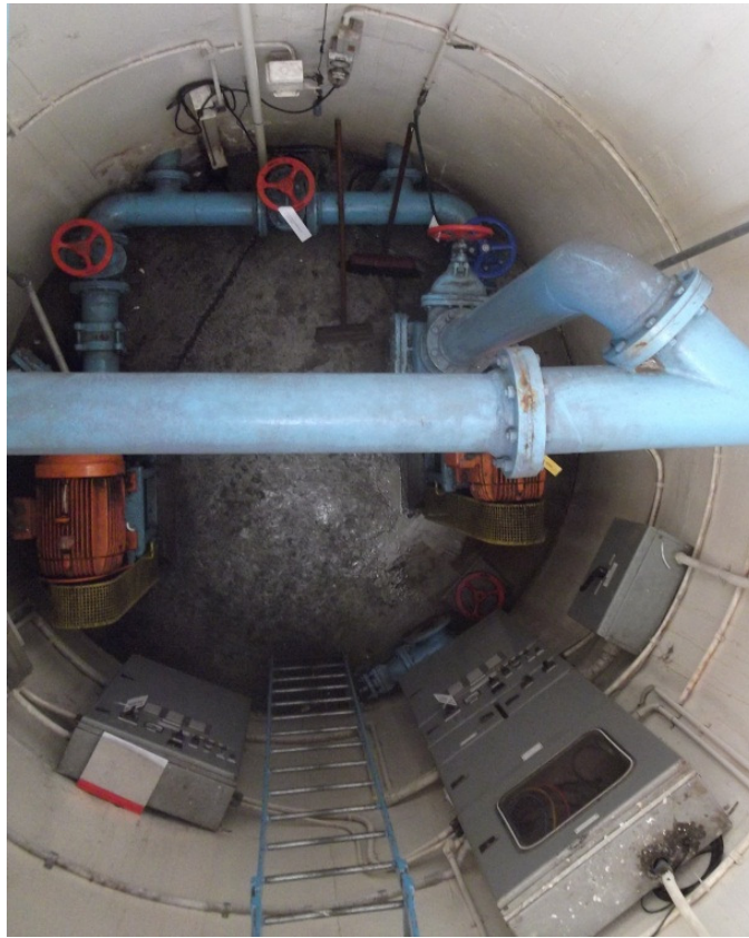
Photo 1 - Pump Station 37 Internal - Existing Layout
