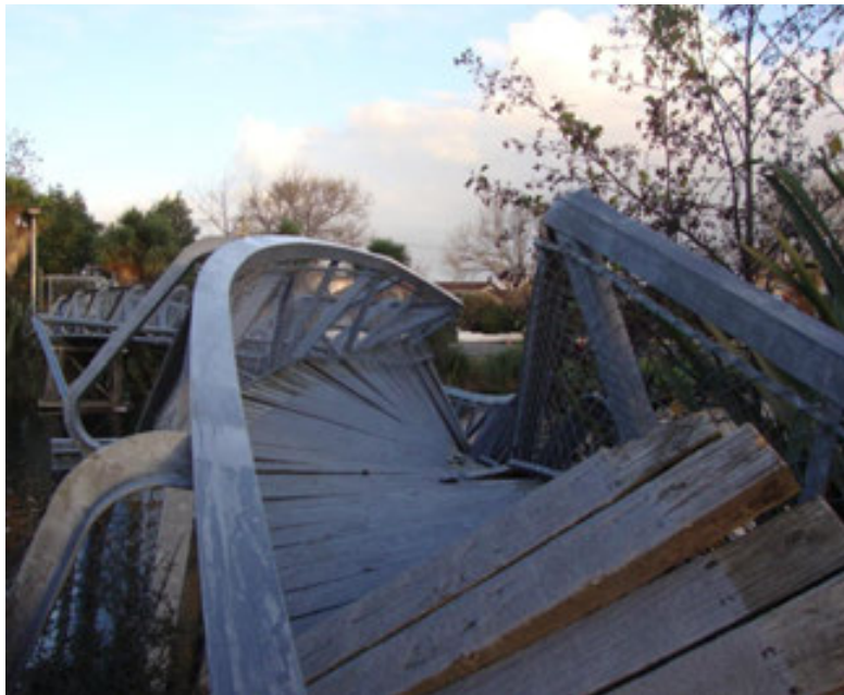
Medway Street Bridge, Christchurch after September 4 th earthquake.
