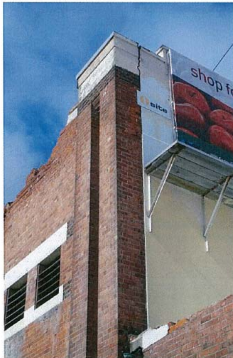
PHOTO 2 – NORTH CORNER SEPARATION AND PARAPET DAMAGE.
