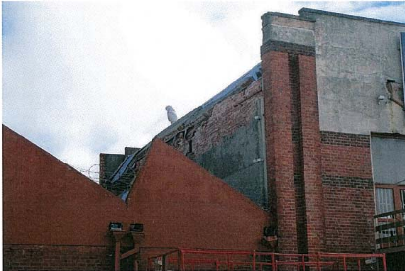
PHOTO 3 – 2 STOREY PART A – SOUTHWEST PARAPET AND WALL DAMAGE. LOSS OF CORNER RESTRAINT TO NORTHWEST AND SOUTHEAST PARAPETS AND WALLS.
