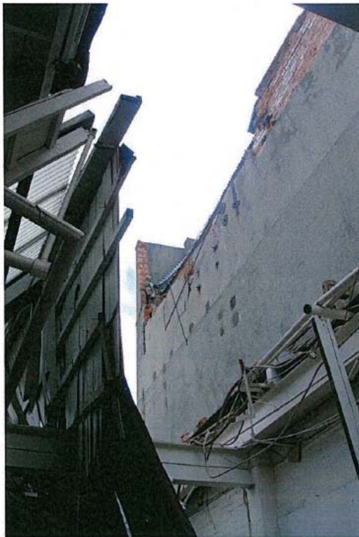
PHOTO 4 – 2 STOREY PART A – SOUTHWEST PARAPET AND WALL DAMAGE. ROOF DAMAGE TO PART C1.
