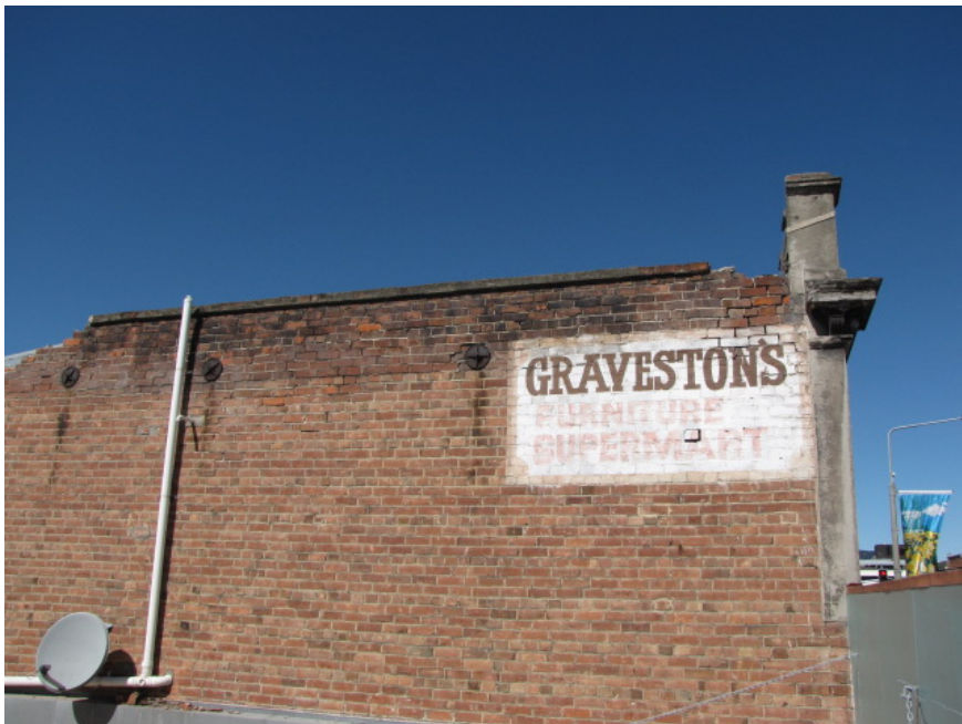
Figure 2: damage to brickwork
