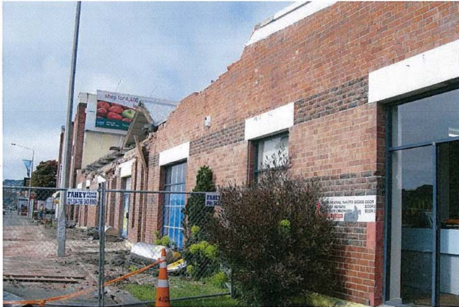
PHOTO 5 – SINGLE STOREY PART B – EXTENSIVE FACADE DAMAGE TO PARAPETS AND WALL. LOSS OF ROOF SUPPORT.
