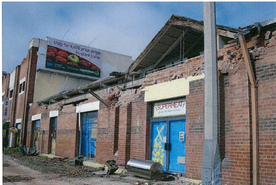
PHOTO 6 – SINGLE STOREY PART B – EXTENSIVE DAMAGE TO PARAPETS AND WALLS LOSS OF ROOF SUPPORT AND TIES TO WALLS
