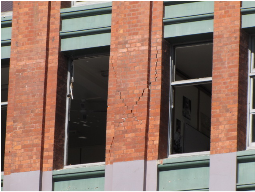
Transverse cracking on north façade
