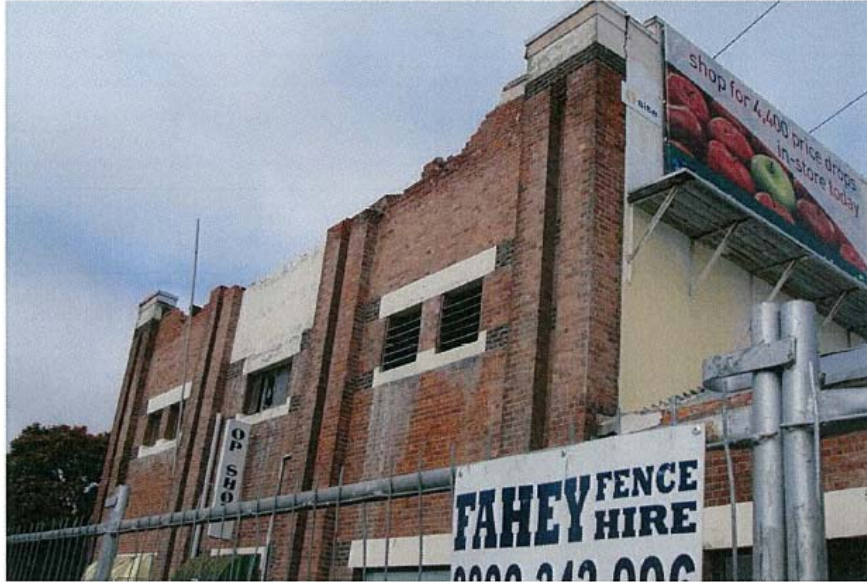
PHOTO 1 – TWO STOREY PART A – NORTHEAST FACADE – EXTENSIVE PARAPET AND WALL DAMAGE.
