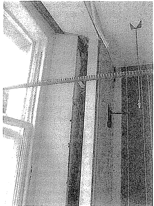
Approx 100mm outward displacement of north wall
