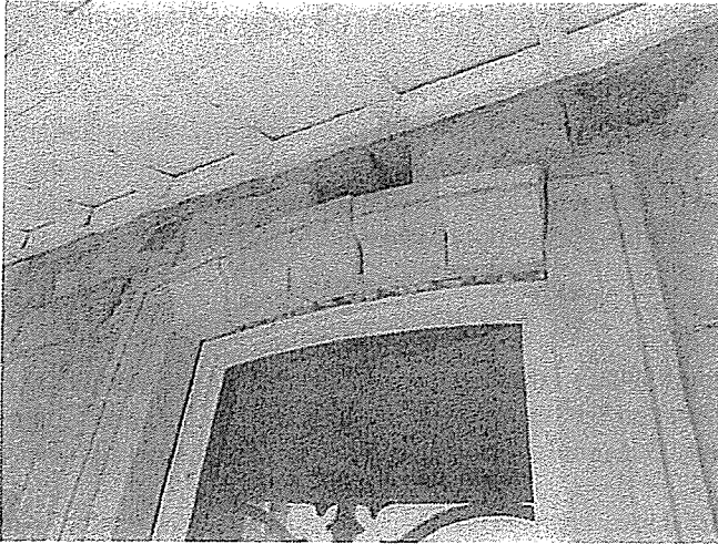
Window lintel arches fell approx 20mm displacing stones above and walls alongside
