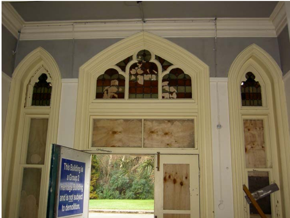
The doorway of the entrance foyer, now secured with plywood over the windows. The toplights feature stained glass. (Photo: J May, 2005 for Conservation Plan, 2006)
