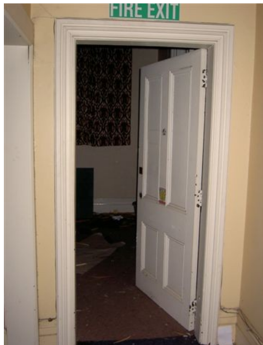
An example of the internal paneled doors. (Photo: J May, 2005 for Conservation Plan, 2006)
