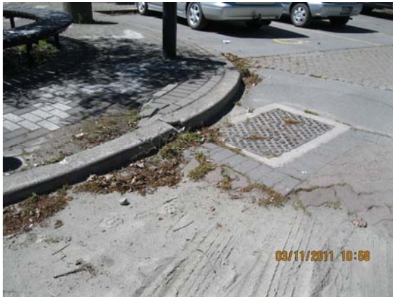
Movements within car park area to West of Building.
