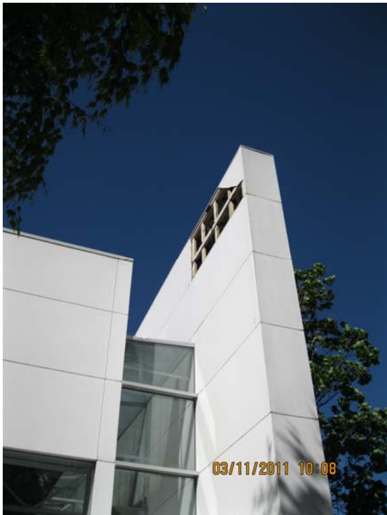
Typical damage to external cladding system.
