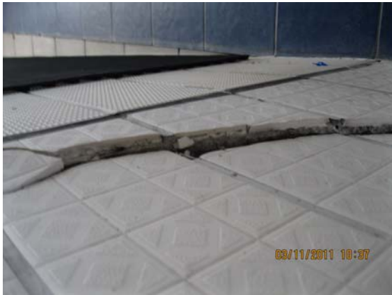
Lifting and cracking of slab along ramp line.
