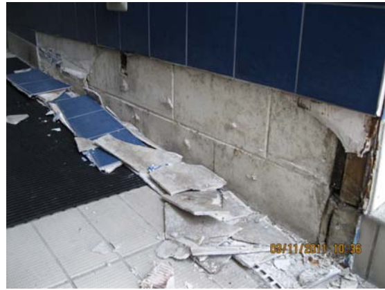
Cracked and delaminated tiles below mezzanine level (a result of differential settlement).
