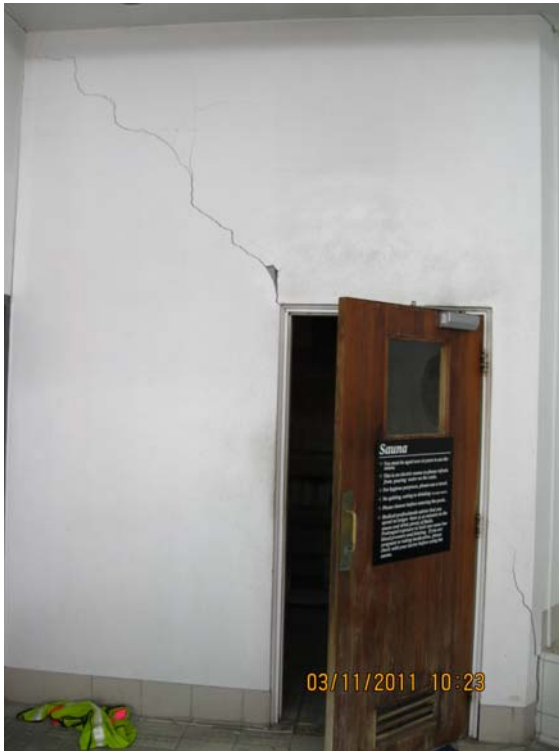
Damage to Blockwork walls (typical).
