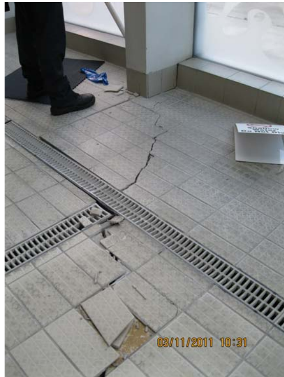
Cracked and unlevel tiling and slab around Gridline 8 (typical).
