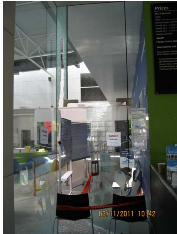
Internal damage to glazing below mezzanine – due to differential settlement.
