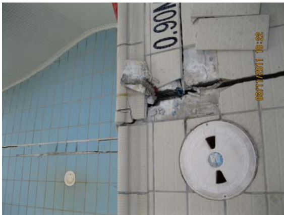
Cracked and deformed pool edge at Leisure pool, levels have dropped across crack extent (typical).
