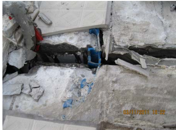
Deformed and widened water stop at edge of main pool (typical).
