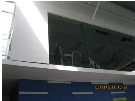
Mezzanine Floor – evidence of deformation and cracking where floor has dropped.
