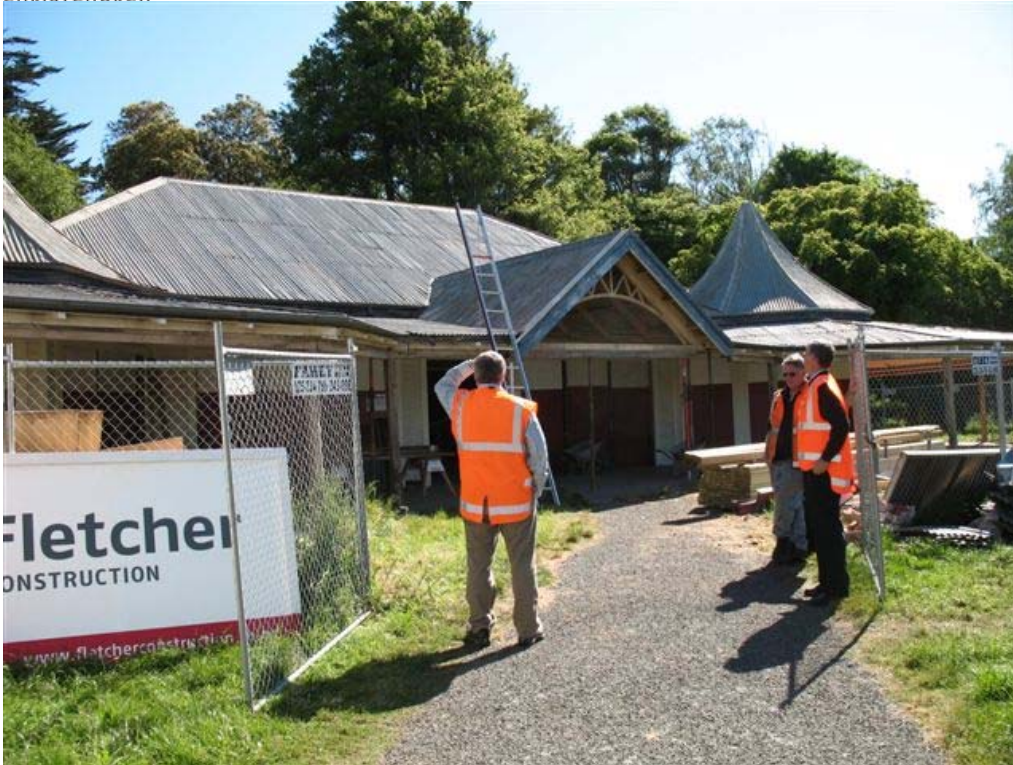
December 2006 – work has ceased at this point awaiting grant monies to continue
