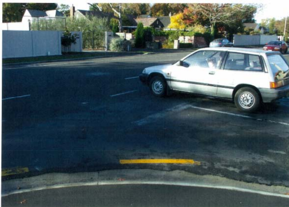
Photo 1 - Faded limited line at the intersection of Hamilton Ave and Clyde Road
