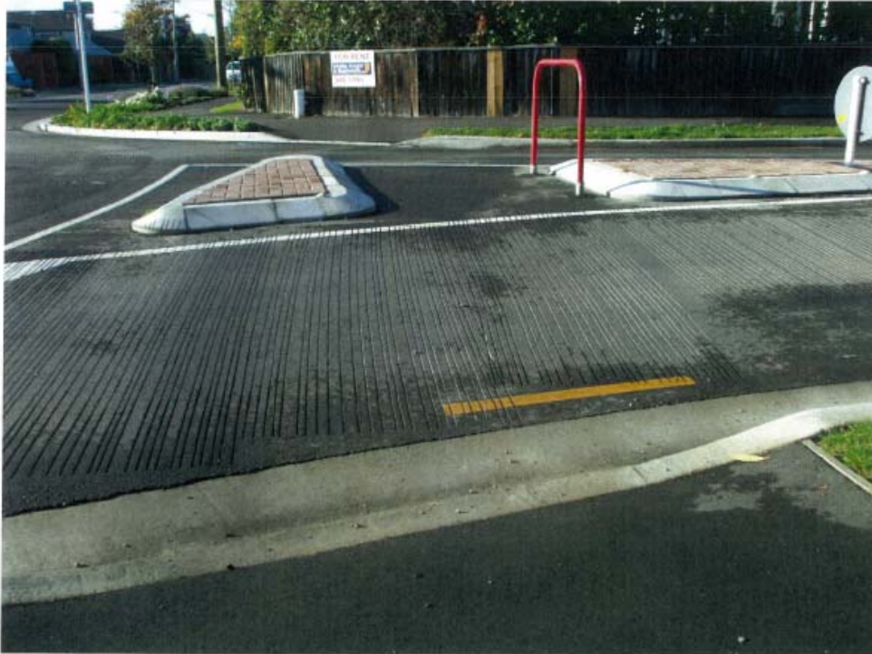
Photo 3 - Incorrect alignment with the crossing direction on Coldstream court
