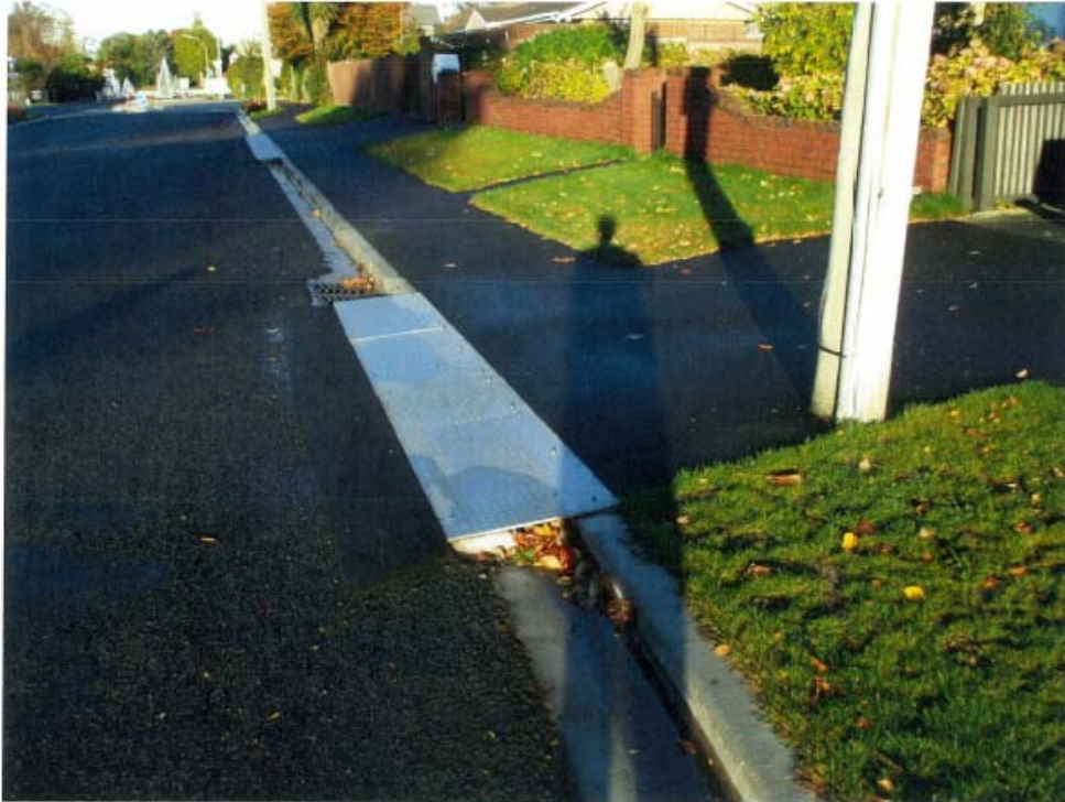
Photo 2- Restricted flow of stormwater in the kerb and flat channel
