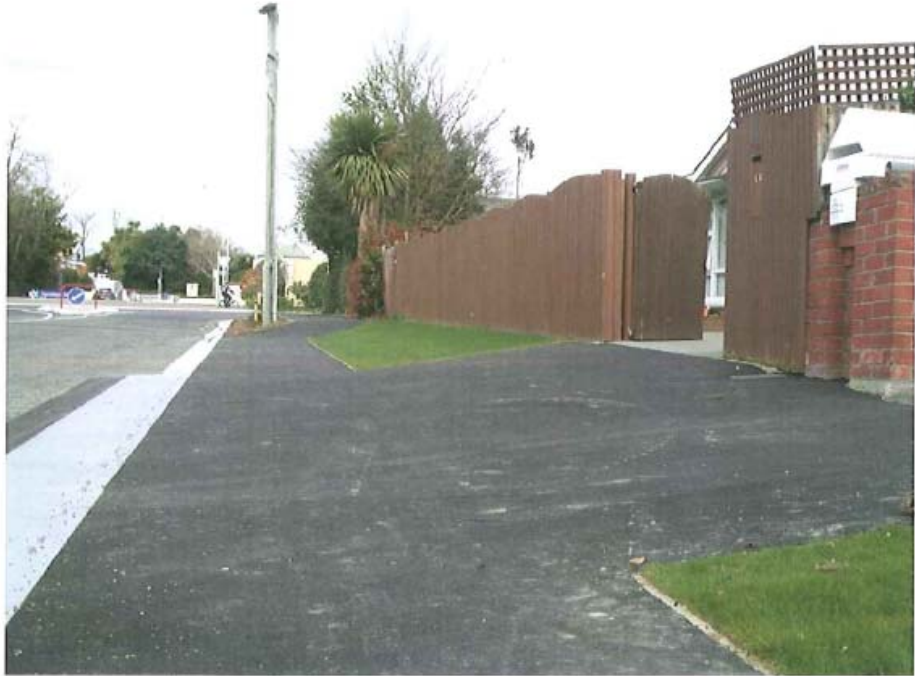
Note how the profile between kerb and property boundary changes as the footpath shifts from the property boundary to the kerb.
