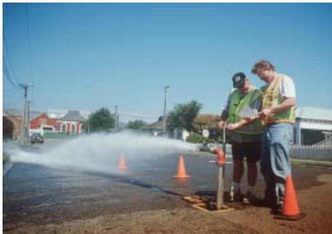
City Care staff testing fire hydrant water pressure.
