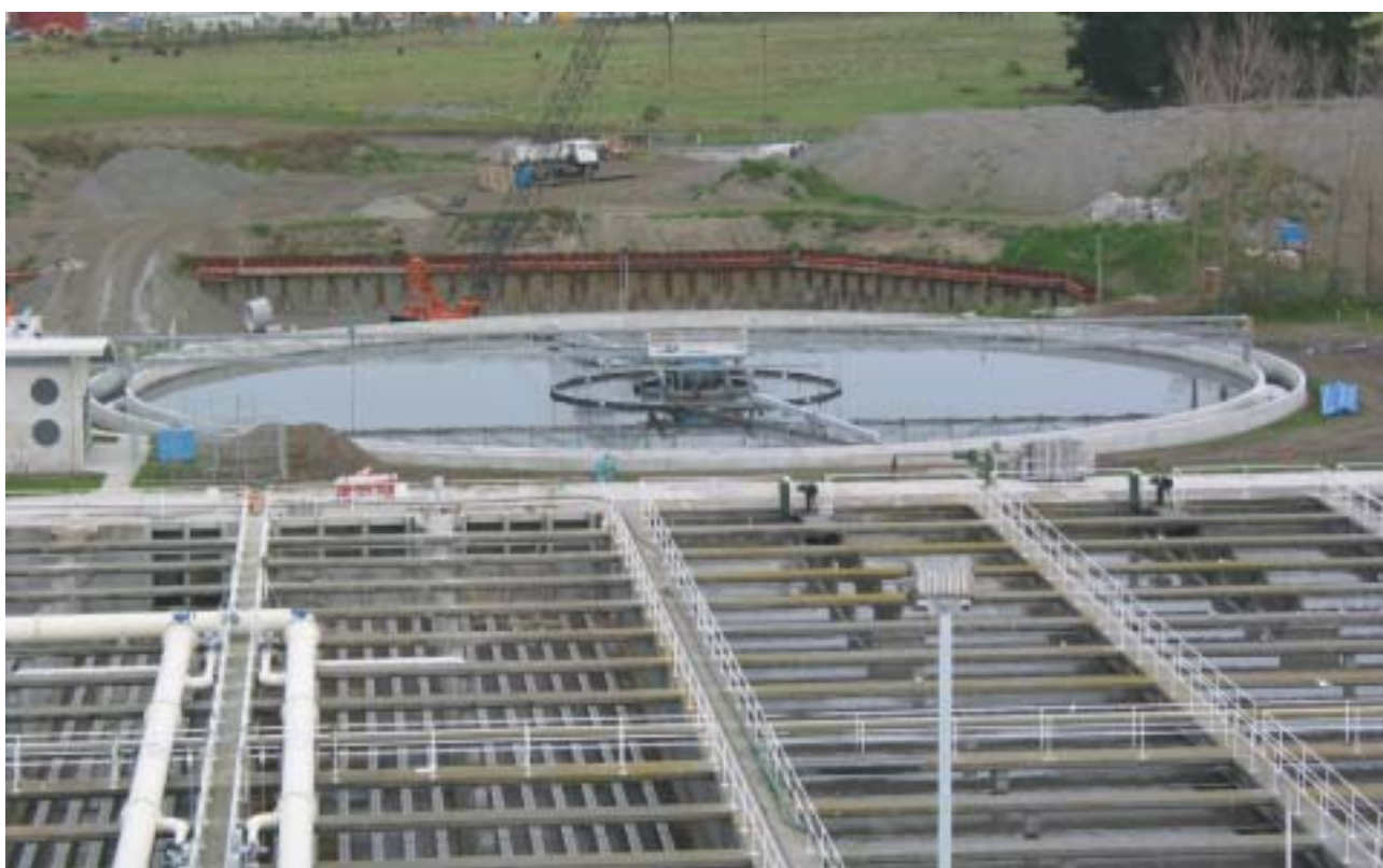
Construction of one of the new clarifiers at the Christchurch Wastewater Treatment Plant.
