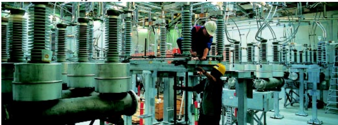
Construction work on Orion's upgraded Armagh Street substation that was completed in 2001
