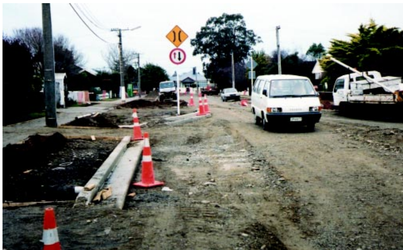
City Care staff working on the Prossers Road kerb and channel renewal and landscaping contract
