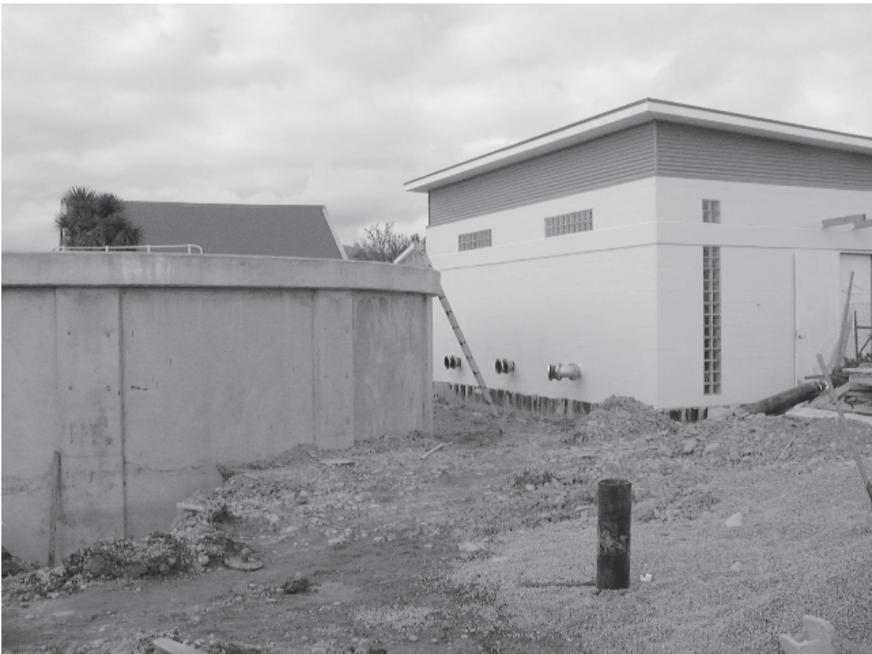
Construction of a new pump station and reservoir at Glenroy St, Woolston. The new pump station, reservoir and wells were completed in January 2001 as part of the Council's ongoing replacement programme, to replace the original station built in 1927.
