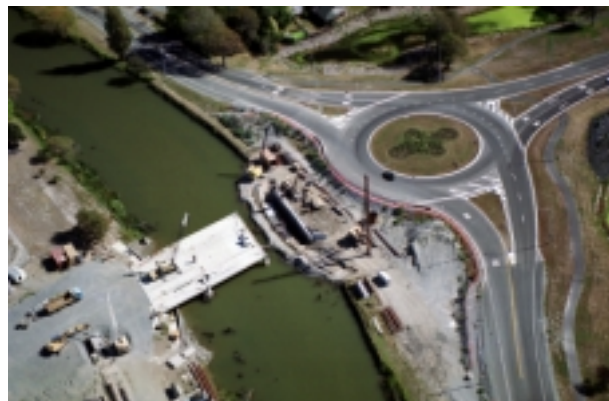
An aerial view of work in progress on the Woolston Burwood Expressway
